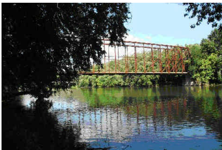
Dearborn County - The Laughery Creek Bridge in Dearborn County is an example of a triple intersection Whipple truss bridge. Commonly referred to as the Triple Whipple, this is the only example known in the United States.
